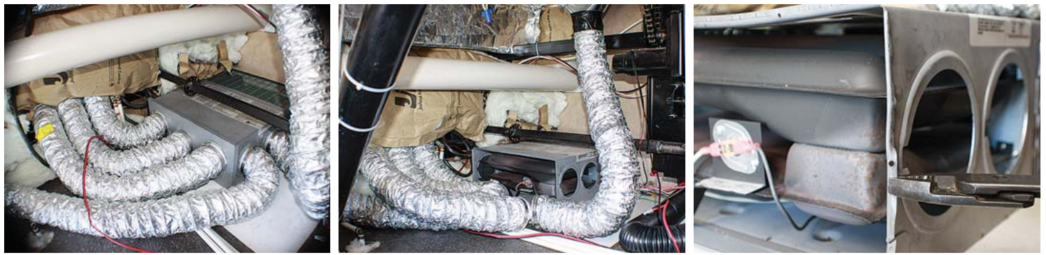
(Above, from left to right) Flexible ducting is routed from six ports in the stock Suburban furnace in the test fifth-wheel. The ducting and collars are removed from the rear panel of the furnace to start the installation process. On this Suburban furnace, pliers were used to fold the tabs flat on both sides of the furnace to allow the new plenum to fit properly.
