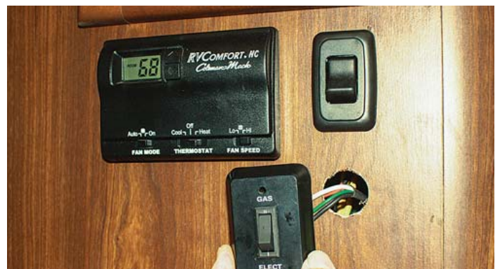
The gas/electric selector switch was mounted in the panel that also housed the existing dual thermostat.
