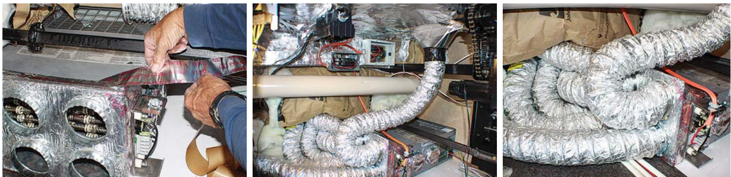
(Below, from left to right) After the heating element is installed into the plenum, the plenum is installed to the rear of the furnace and high-temperature aluminum foil tape is used to seal the edges. At the top the junction box for the 50-amp service is installed. Below is the disconnect switch, and to the right the system controller is mounted. The orange, 10-gauge Romex runs between the J-Box to the disconnect switch to the controller then runs down to the heating element. The flexible heat ducting is attached to the plenum.
